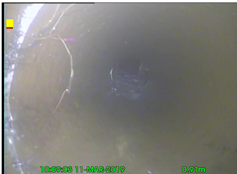
Photo: 4_4a, 00:00:00 0.91m, Fine Roots at joint , from 09 to 11 o'clock
