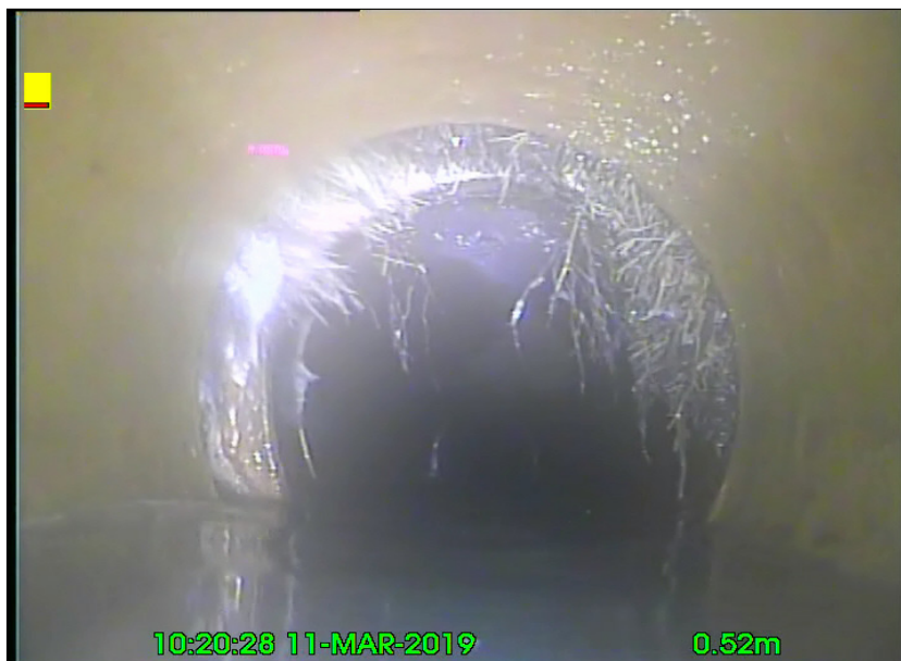
Photo: 13_5a, 00:00:00 0.52m, Fine Roots at joint , from 07 to 05 o'clock
