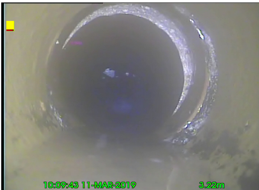
Photo: 8_8a, 00:00:00 3.22m, Joint displaced medium
