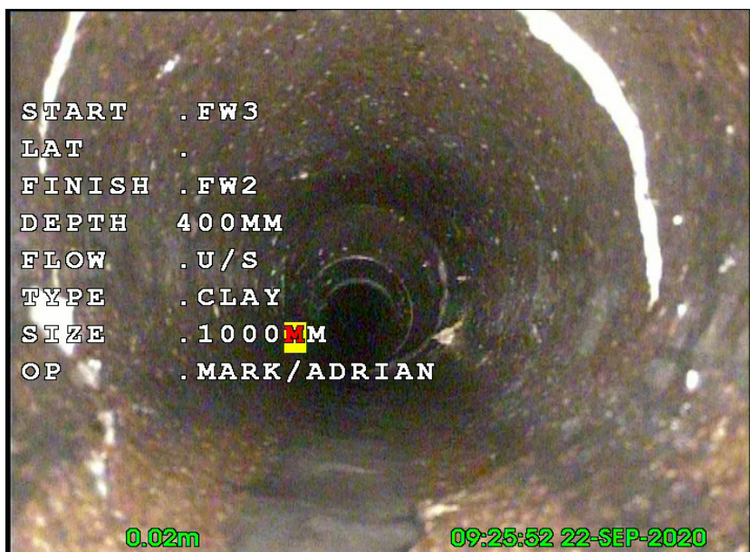
Photo: 22_3a, 00:00:00 0.02m, Fracture Circumferential from 08 to 04 o'clock
