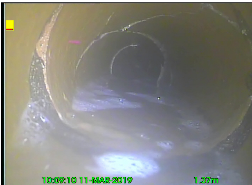
Photo: 6_6a, 00:00:00 1.37m, Fractures multiple from 08 to 03 o'clock
