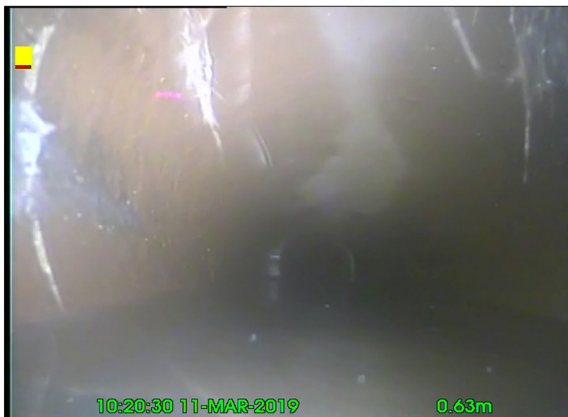
Photo: 15_6a, 00:00:00 0.63m, Crack Circumferential from 07 to 11 o'clock
