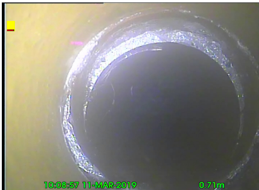
Photo: 3_3a, 00:00:00 0.71m, Joint displaced medium
