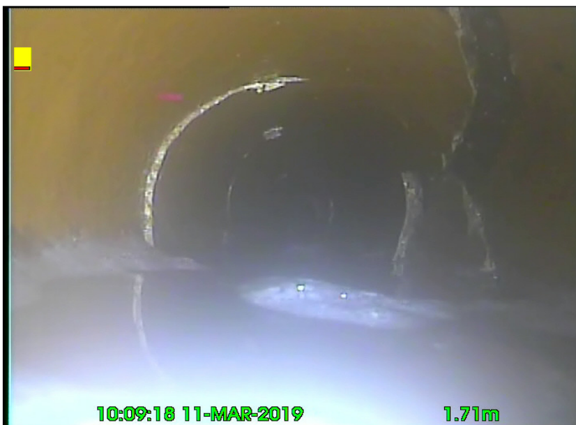
Photo: 7_7a, 00:00:00 1.71m, Hole in sewer from 01 to 05 o'clock
